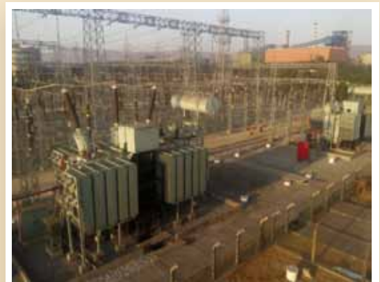
Electrical Projects Division commissioned the 220kV Substation at Hospet, Karnataka
